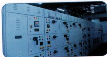
Electrical Turnkey Project
