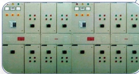
APFC Control Panel
